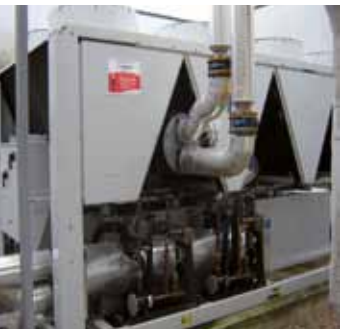
The cooling unit of the heat pump at the Pasteur Clinic in Royan, France.
