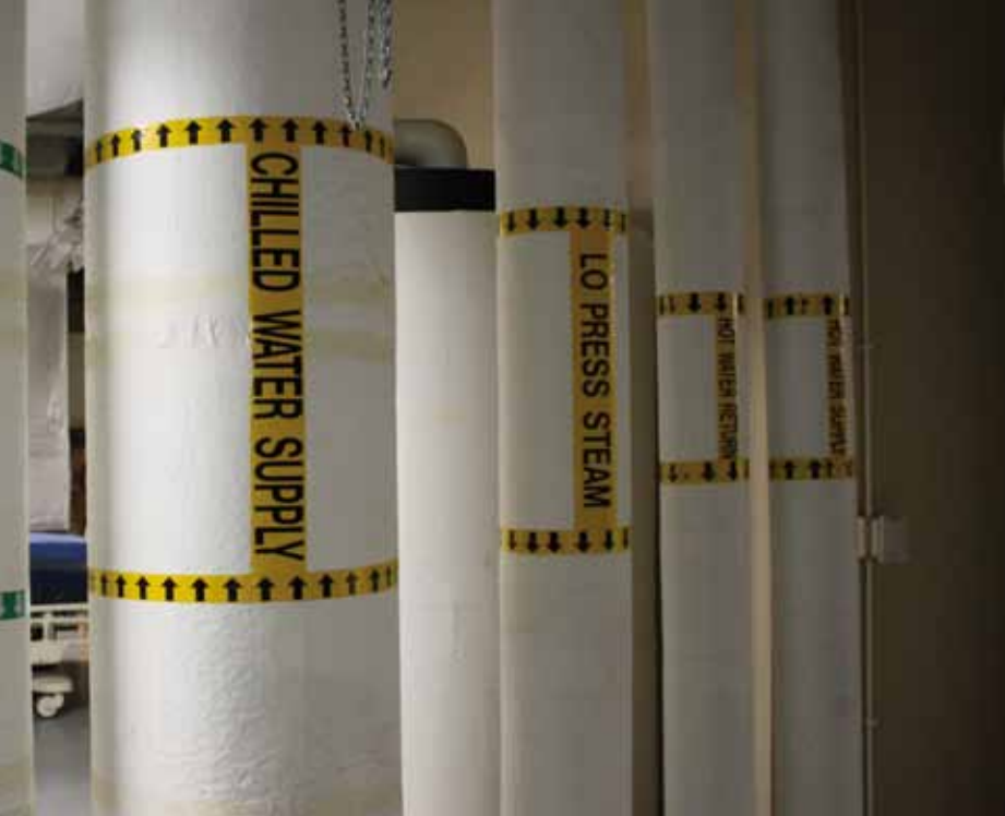
The refrigeration system of the Fletcher Allen Hospital in Burlington, Vermont, USA.
