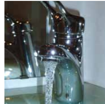
Eco-aerator at the Navarre Polyclinic in Pau, France.
